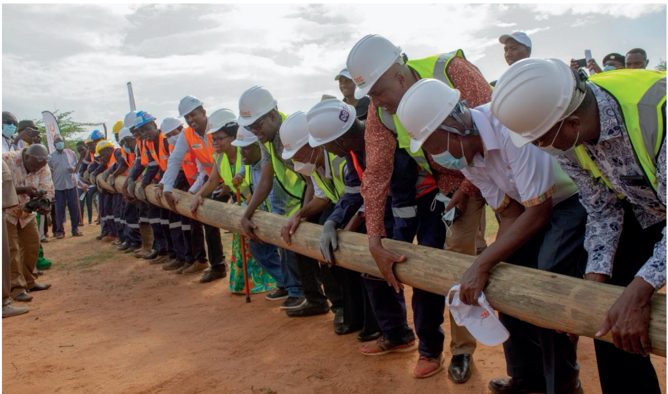
REREC officials and engineers erecting electric pole at Wekoye Primary School during the Corporation’s ground-breaking ceremony for EPFP in Tana River County. The project aims to connect to power over 1,200 public facilities and over 35,000 households across the country by June 2022.
